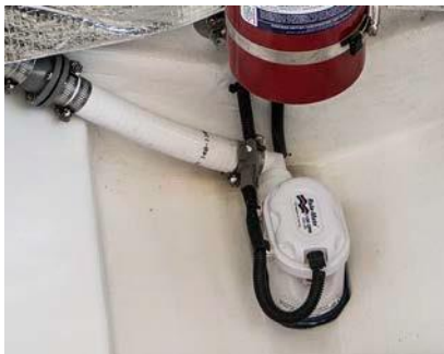
Aft BILGE PUMP
