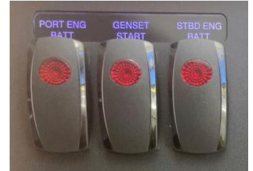
Engine Battery Switches
