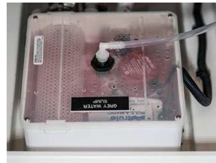
GRAY WATER SUMP
