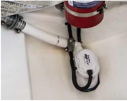
Aft BILGE PUMP
