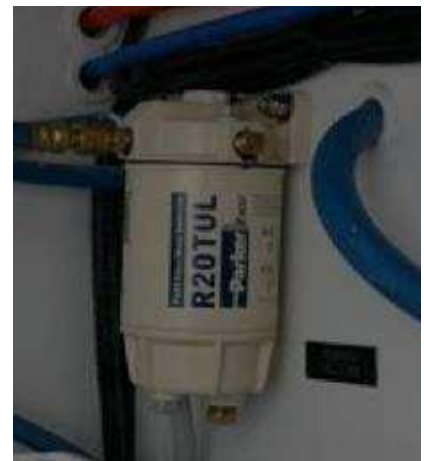
GENERATOR FUEL PRE-FILTER is behind the generator against the bulkhead
