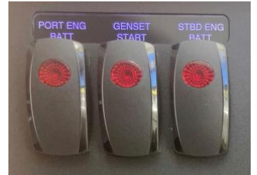
Engine Battery Switches
